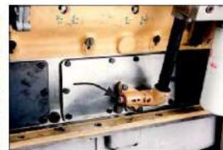
V-28 Coolant drain point
