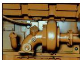
KTA-3007 Coolant drain point
