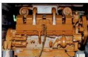
KTA-2500 Coolant drain point
